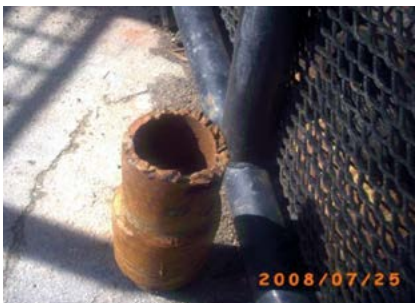
Broken HDD drill stem pipe
