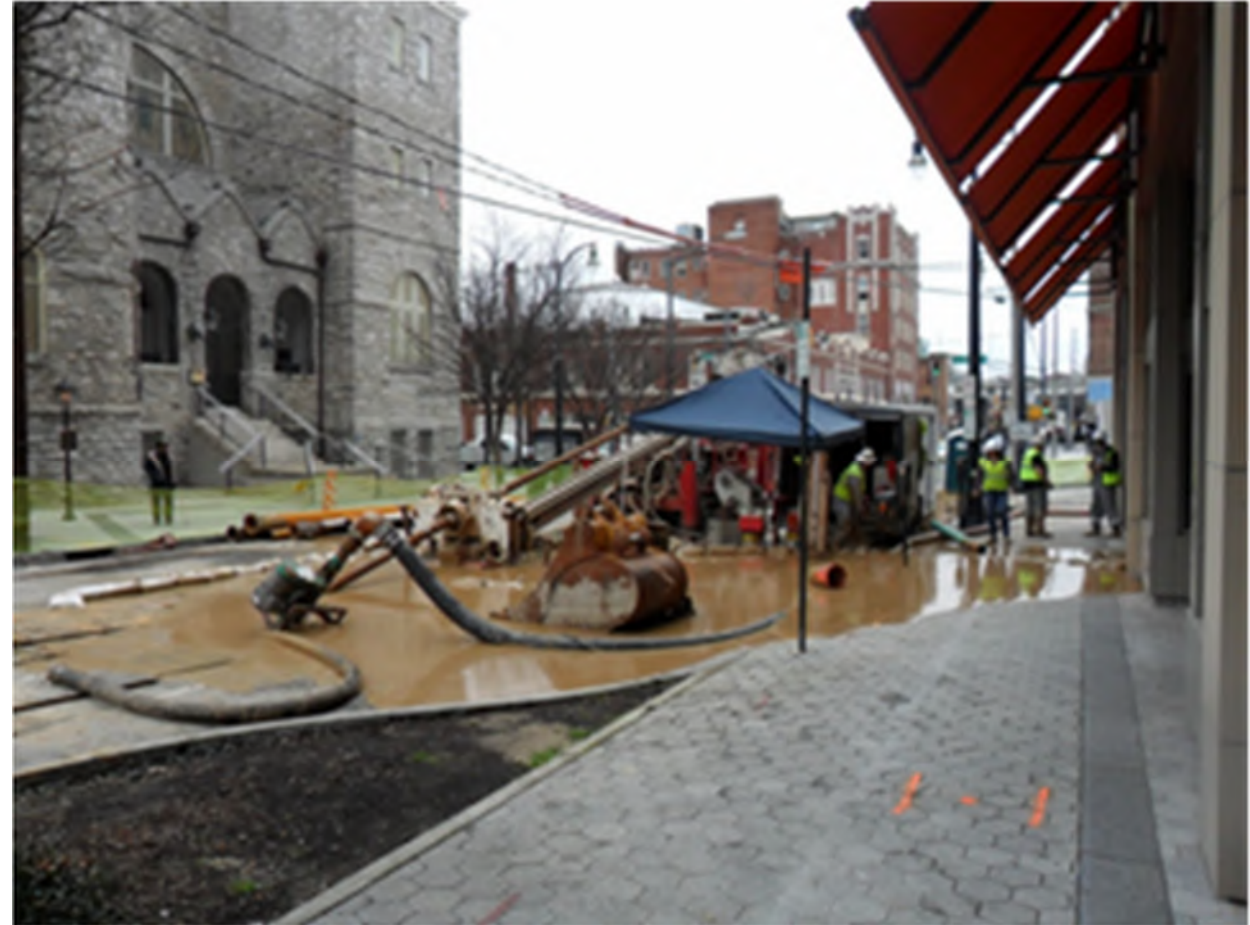
"Backflush" event during pilot hole drilling flooded street with 15,000 gallons of groundwater. "Pocket of water" on shallow, denser rock surface was recharged by rainfall.
